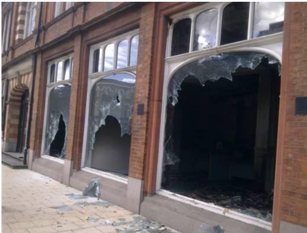
Damage to 639 High Road
